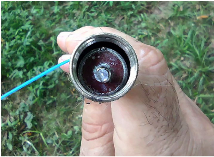
Corrosion produced by water seeping into coax connector (Image by author)
